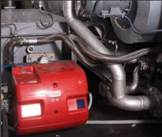
Gas Heating System
